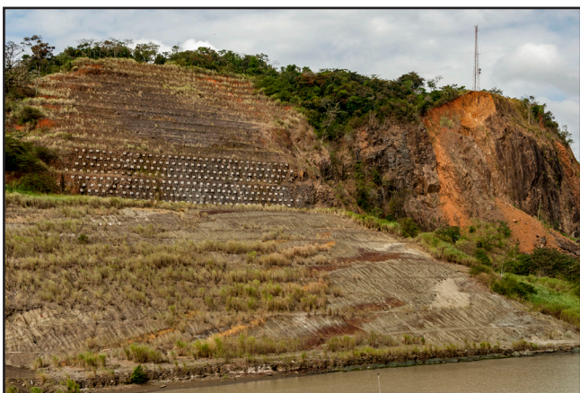
Figure 15. The cut face of Zion Hill in the Culebra Cut; the terraced face in the Pedro Miguel volcanic rocks is constrained by 250 rock anchors to prevent it from sliding out over the underlying Cucaracha Clay that has been cut back to a gentle profile.
